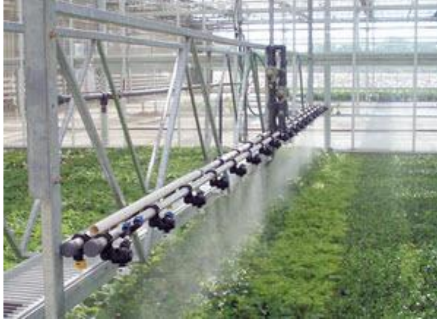
Figure 1.4 Custom design of a humidifier system for a greenhouse [41].
